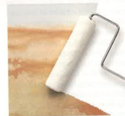
● Blocking water stains.
